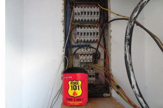
Indoor Electric Board
