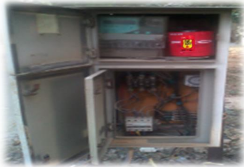
Outdoor Electric Board
